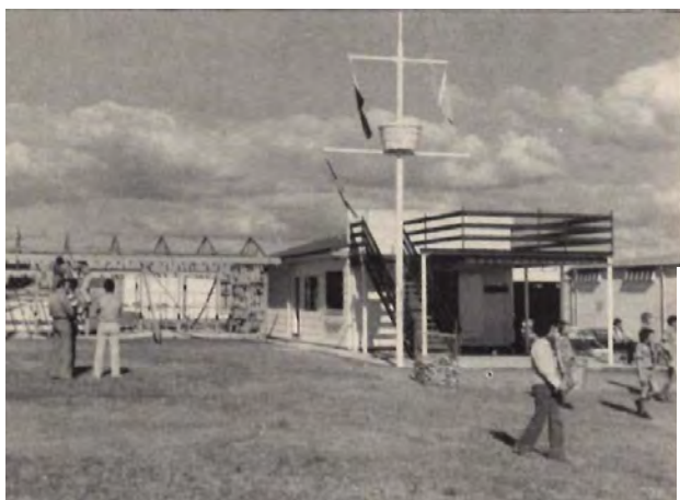
The Scout Activities building,, later named the Raoul Mondon Hut under construction
